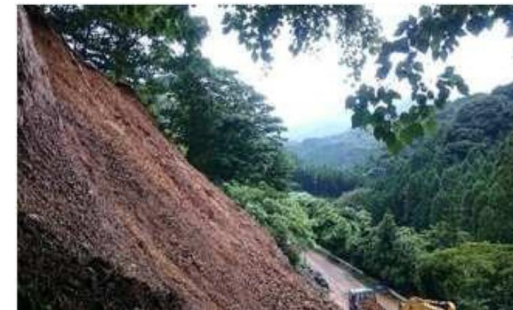
Figure 7.3.10 Photo After Damage to the Cut Slope of the Road
