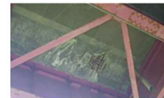
(c) Delamination and rebar exposure
