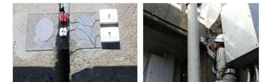
Sensor Installation Status
