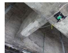
Sensor Installation Status
